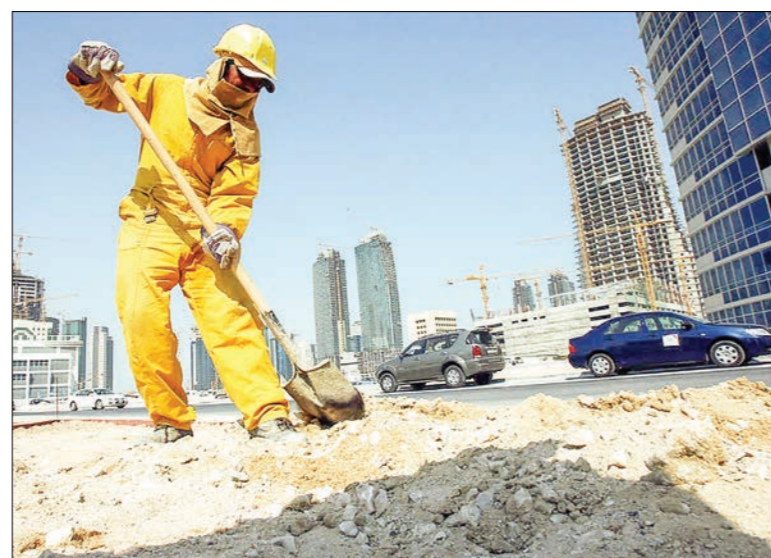
A construction worker digs at a building site while in the background numerous cranes are positioned around high-rise apartment buildings under development in the Qatari capital Doha. PHOTO: AFP
