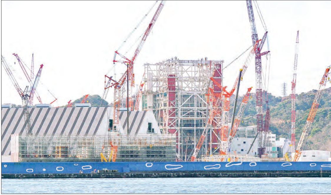
File photo taken in February 2021 shows a coal-fired power plant under construction in Yokosuka. PHOTO: KYODO NEWS
