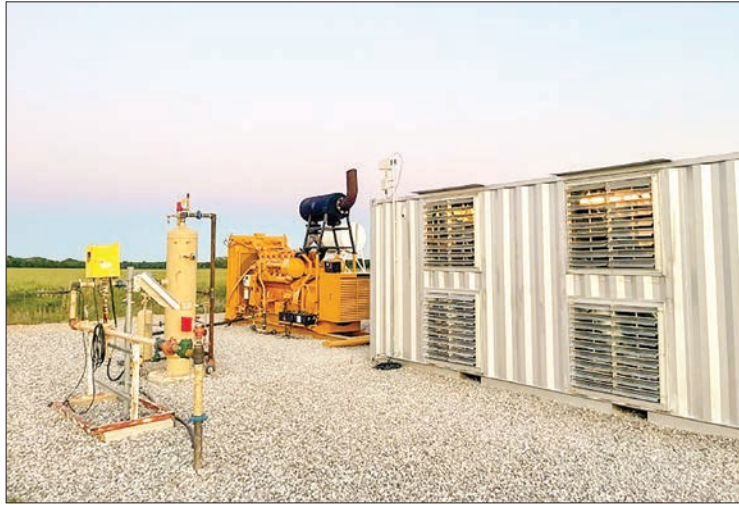
A handout photo from Giga Energy Solutions shows a natural gas generator powering a bitcoin mining center in north Texas in May 2021. PHOTO:AFP
