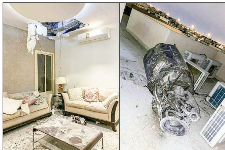
Damage to a home and debris on the roof of a building in Saudi Arabia’s capital Riyadh in the aftermath of a missile attack claimed by Yemen’s Huthi rebels in February 2021. PHOTO: AFP
