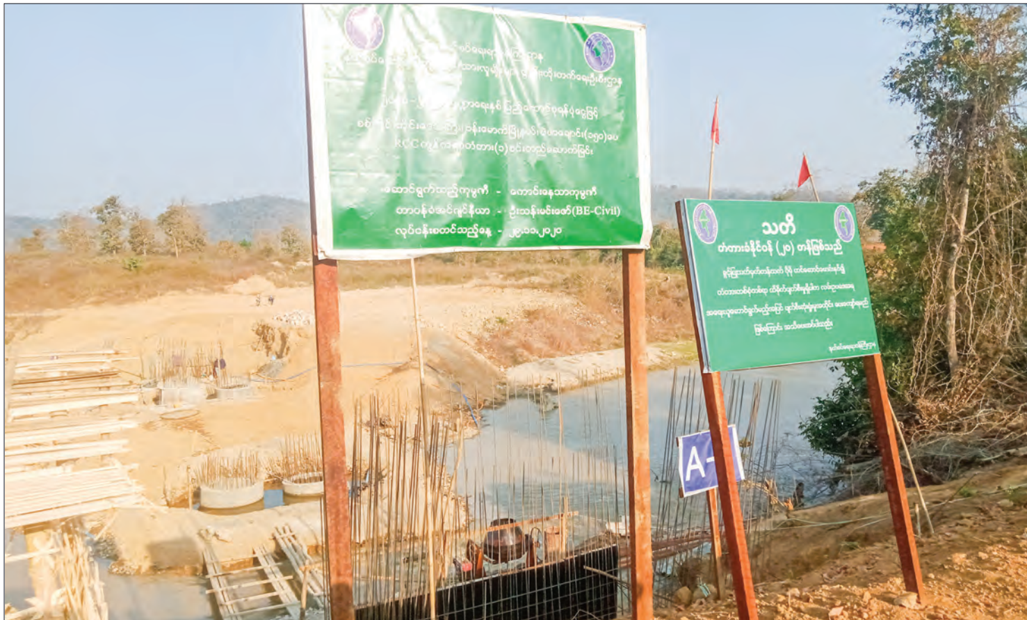
Now, the Kawpok-creek-crossing bailey bridge is being constructed in Bamauk Township. PHOTO: KHIN MAUNG SWE (MAW LUU)
