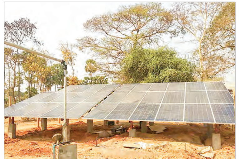
An entirely-completed solar water supply system is seen in Magway. PHOTO : THAN LWIN (MAGWAY)
