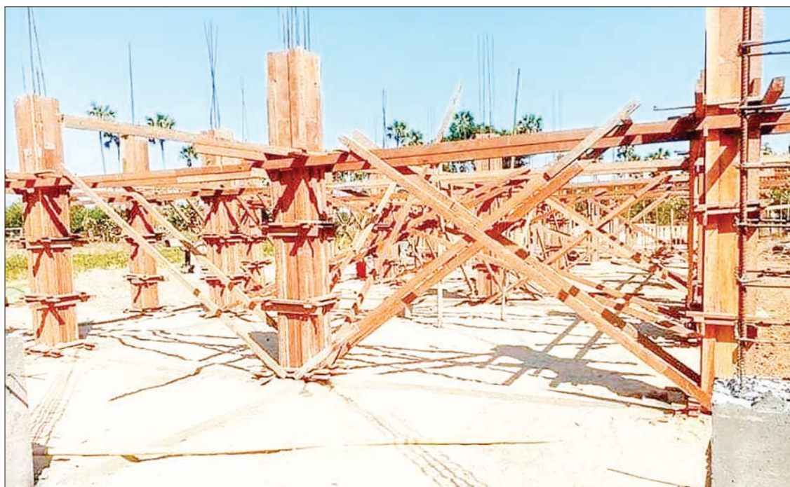
The school shelter building started its construction, with a spending of over K140 million from the National Natural Disaster Management Committee's fund of the 2020-2021 financial year.
