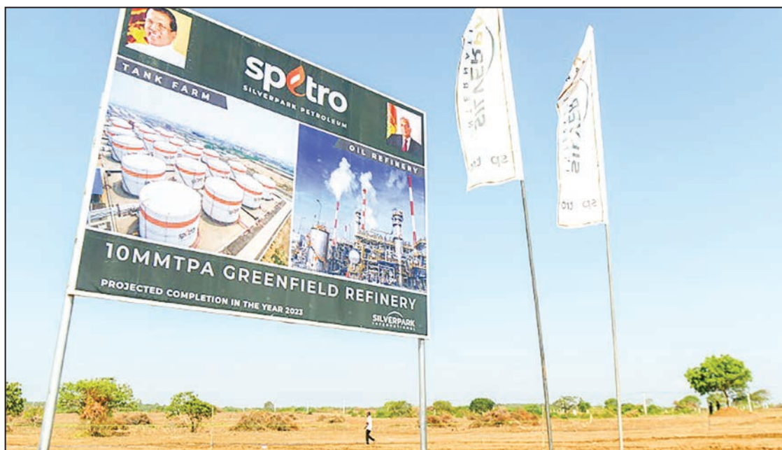
An oil refinery facility under construction at Hambantota. Sri Lanka was forced to hand over Hambantota port on a 99-year lease to a Chinese firm in 2017 after Colombo said it was unable to service the $1.4-billion debt from Beijing used to build it. PHOTO: AFP
