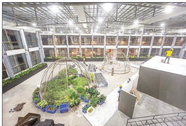
Ongoing construction work at Connect@Changi's courtyard. The facility at Singapore Expo and Max Atria is almost complete and is expected to receive its first guests under the Connect@Singapore segregated travel lane from Feb 21. PHOTO: CONNECT@CHANGI/FACEBOOK
