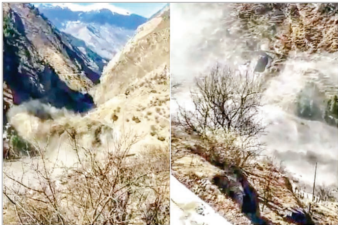
A rescue operation to clear Tapovan tunnel from debris following floods. PHOTO: INDO TIBETAN BORDER POLICE HANDOUT/AFP
