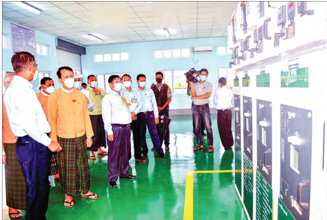
Yangon Region Chief Minister U Phyo Min Thein inspects the Aikalaung power substation in Taikkyi Township, Yangon Region on 31 January 2021. PHOTO: MIN HTET
