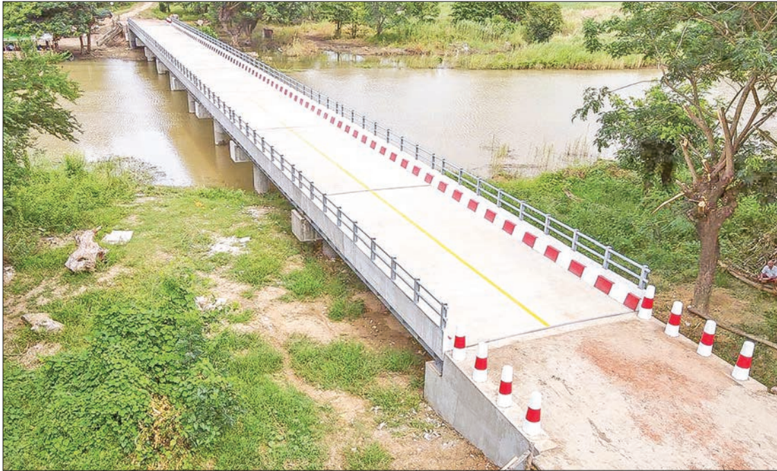
Picture shows the newly-opened Ngar Kyee Bridge in Monyo Township, Bago Region. PHOTO: TIN SOE (BAGO)
