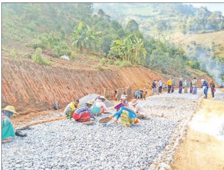
Authorities inspect the progress of Lat Taing-Pan Un road construction near Na Khaik/Na Than Village-Tract, Hsihseng Township.
