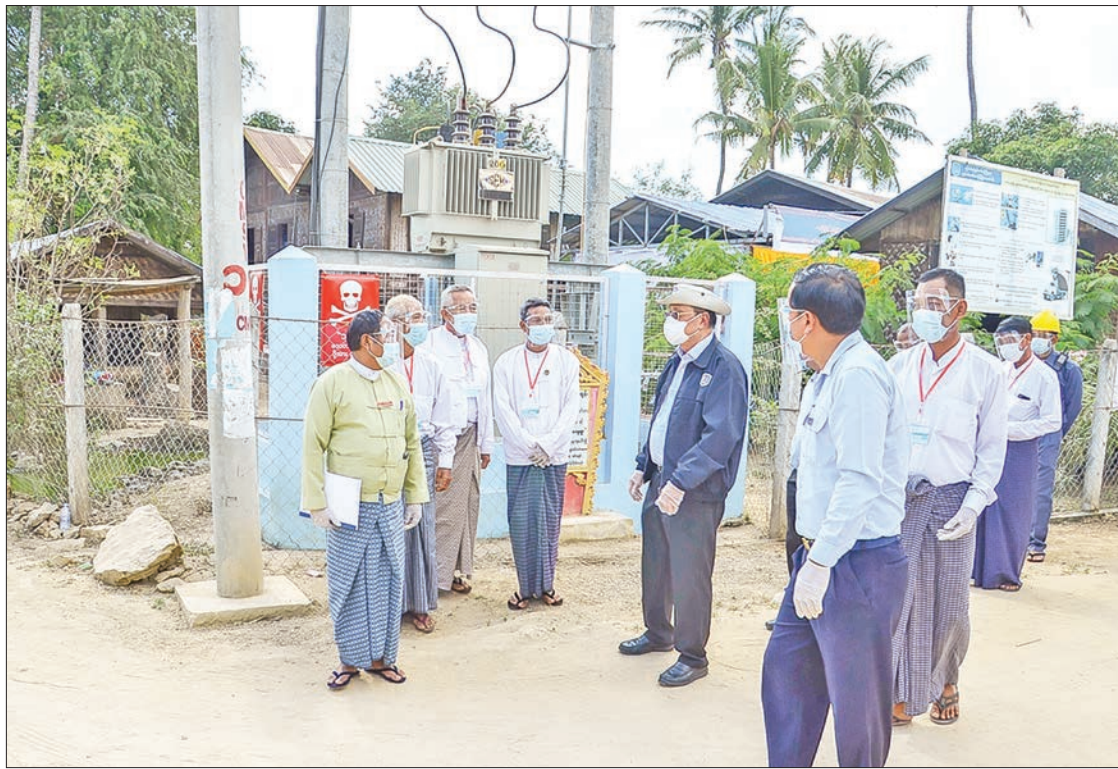
Union Minister U Win Khaing and party visit Shar Taw Village electrified by National Electrification Plan (NEP) in Tatkon Township, Nay Pyi Taw on 5 December 2020. PHOTO: MNA
