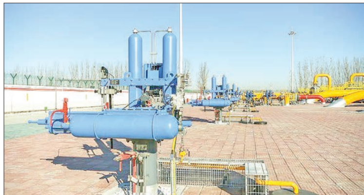
Photo taken on Dec. 3, 2020 shows the Yongqing compressor station of the Changling-Yongqing section of the China-Russia east-route natural gas pipeline in Yongqing County, north China's Hebei Province. The China-Russia east-route natural gas pipeline's Changling-Yongqing section, linking Changling of northeast China's Jilin Province and Yongqing of north China's Hebei province, went into operation on Thursday. PHOTO: XINHUA
