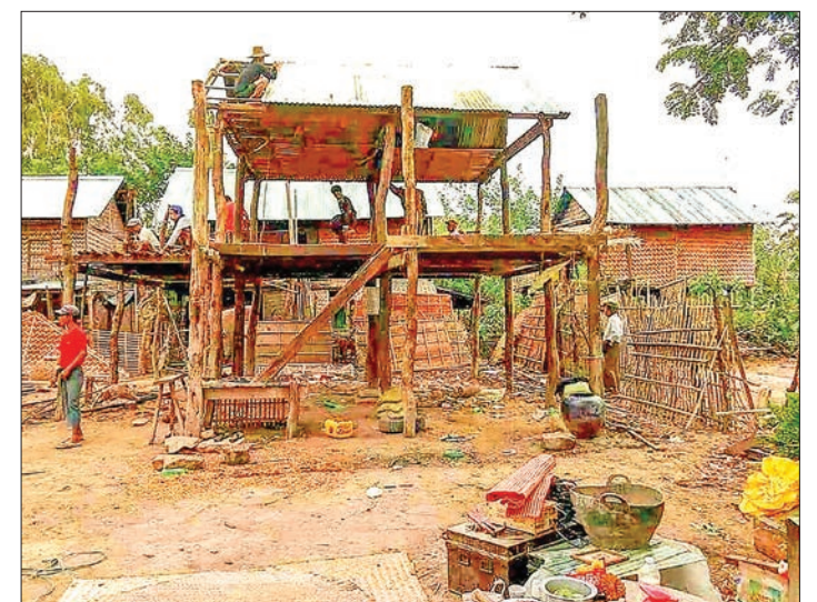
Residents rebuild the house damaged by strong winds at a village in Magway Region. PHOTO: ZAYYATU (MAGWAY)
