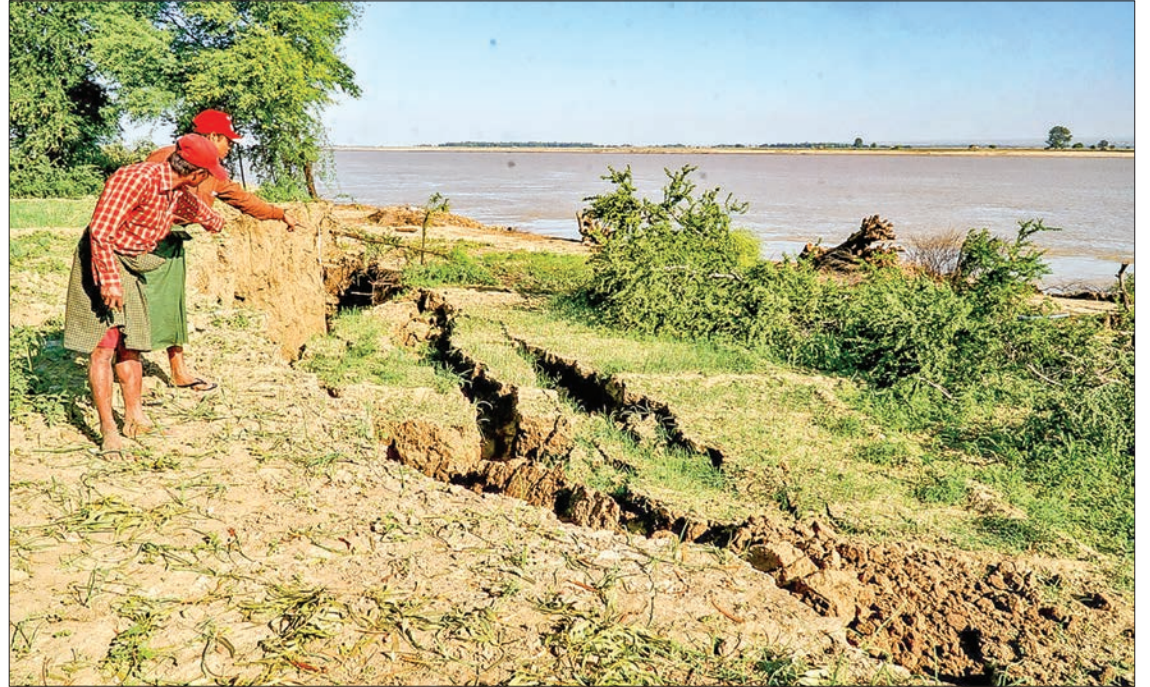
Photo shows the site of the riverbank collapse in Pwintbyu, Magway Region. PHOTO: THAN NAING OO
