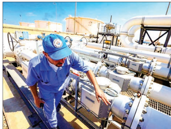
A Libyan oil worker from the Libyan National Oil Corporation checks an oil pipelines at the Zawiya oil installation on 22 August, 2013 in Zawiya, Libya. PHOTO: AFP
