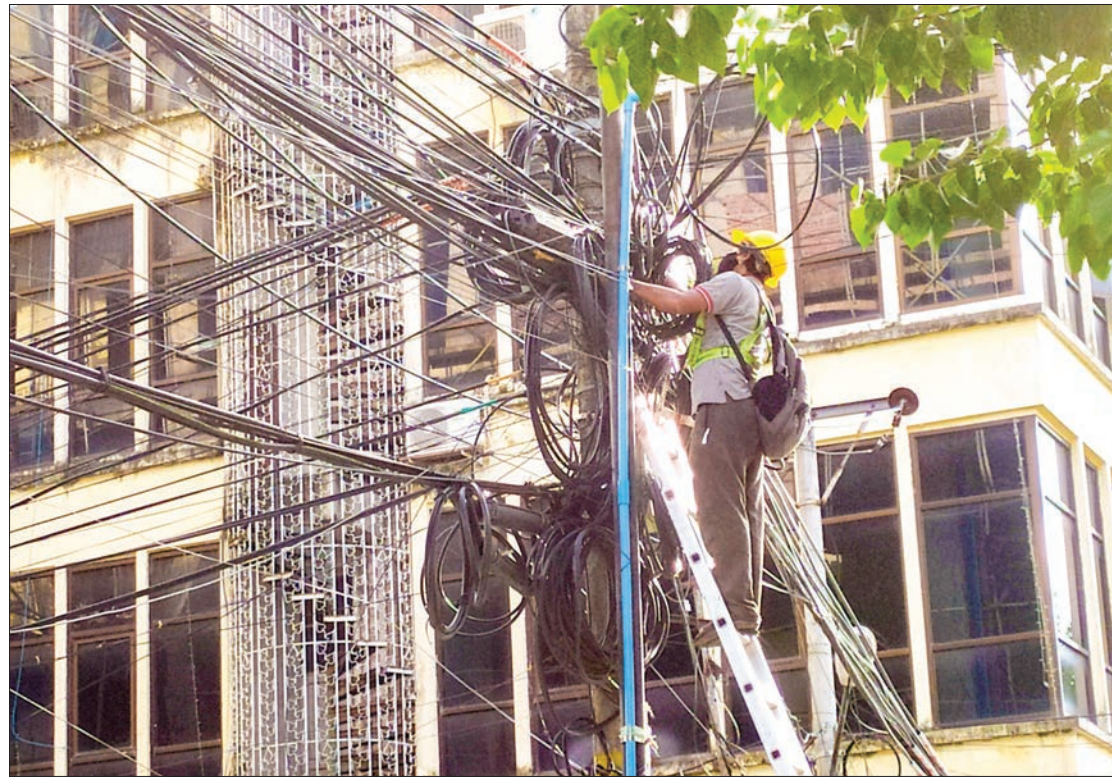
A man carries out maintenance of internet cables at a street lamp post in Yangon on 3 September 2020.
