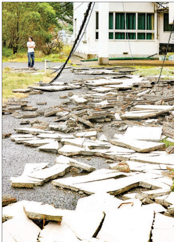
Broken pieces of the exterior wall of a gymnasium are seen scattered on the ground in Nagasaki, southwestern Japan, on 7 September 2020, after they were blown off by strong winds brought by powerful Typhoon Haishen. PHOTO: KYODO NEWS
