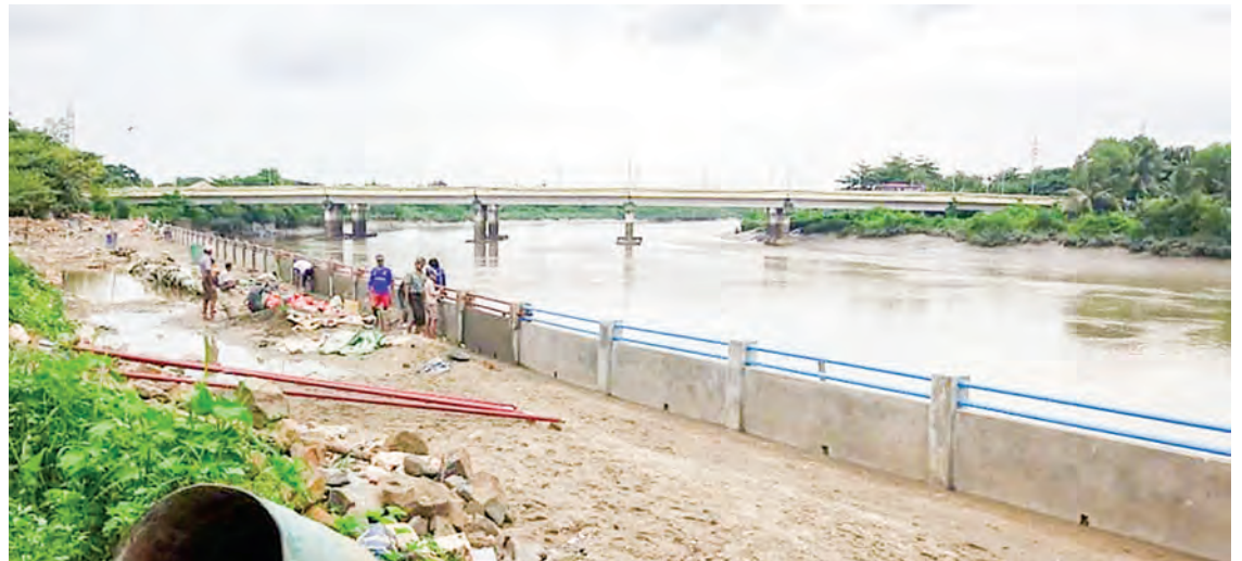
Nga Moe Yeik embankment construction nearing completion in South Okkalapa Township, Yangon. PHOTO: MYINT MAUNG
