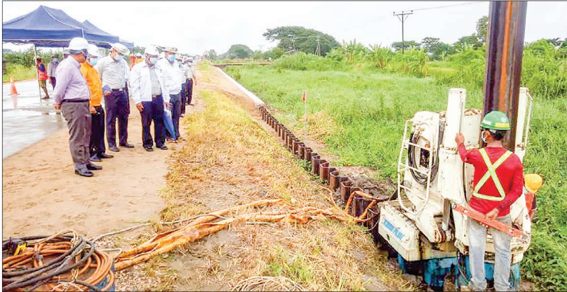
Deputy Minister Dr Kyaw Linn inspecting the repairing works between Yangon and Bo Myat Tun Bridge on Yangon-Pathein road on 23 August 2020. PHOTO: MNA
