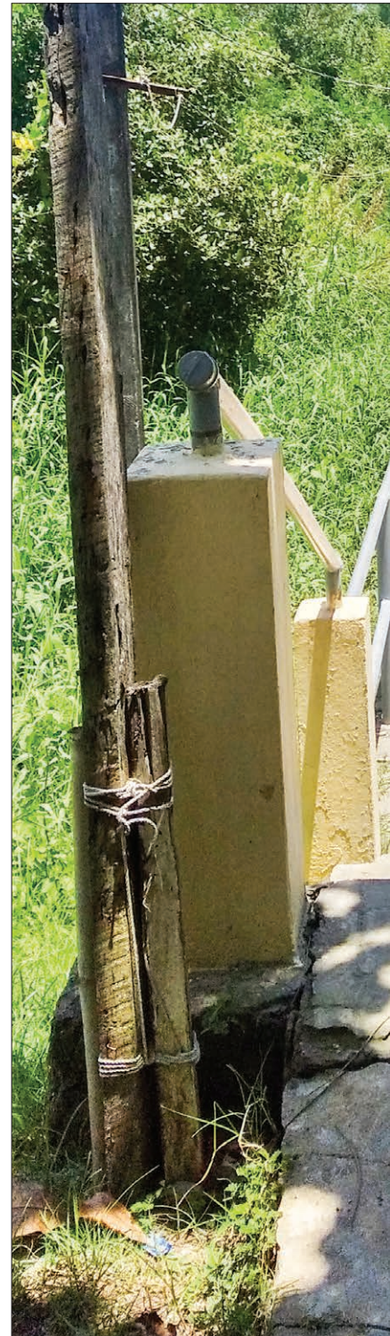
A bridge destroyed by erosion being seen.
