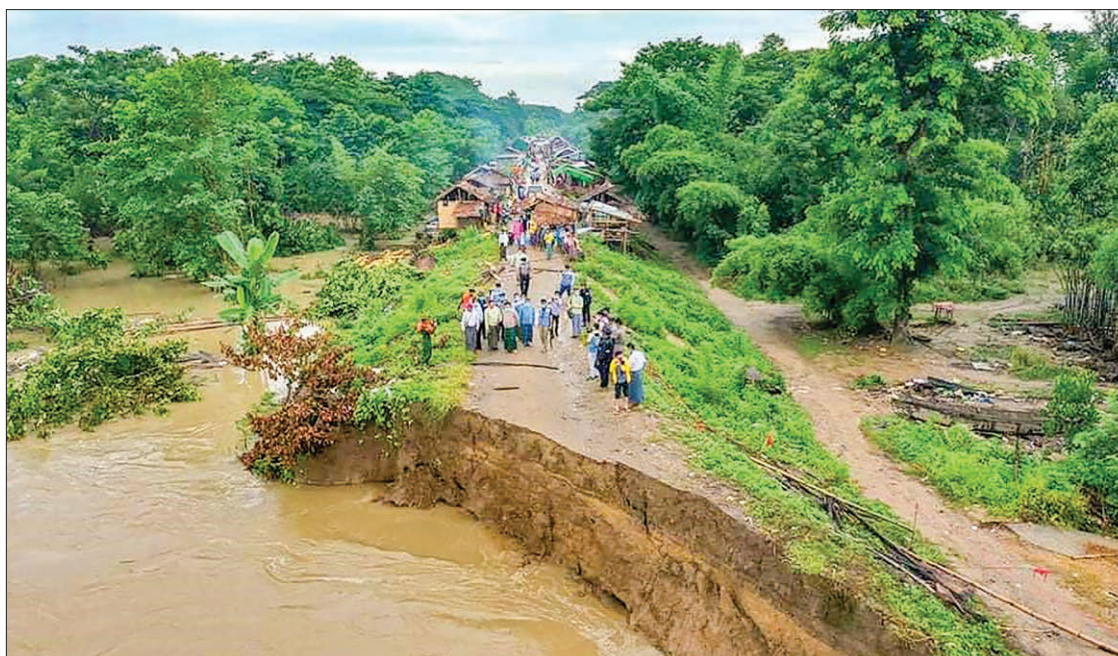
Union Minister Dr Win Myat Aye inspects damages to road caused by flood of Ayeyawady River. PHOTO: MNA
