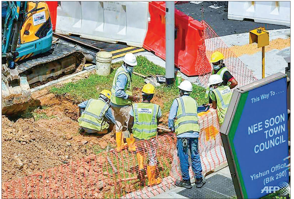
Migrant workers take part in repair work next to a road in Singapore on Jun 3, 2020. (PHOTO: AFP/ROSLAN RAHMAN)/FILE
