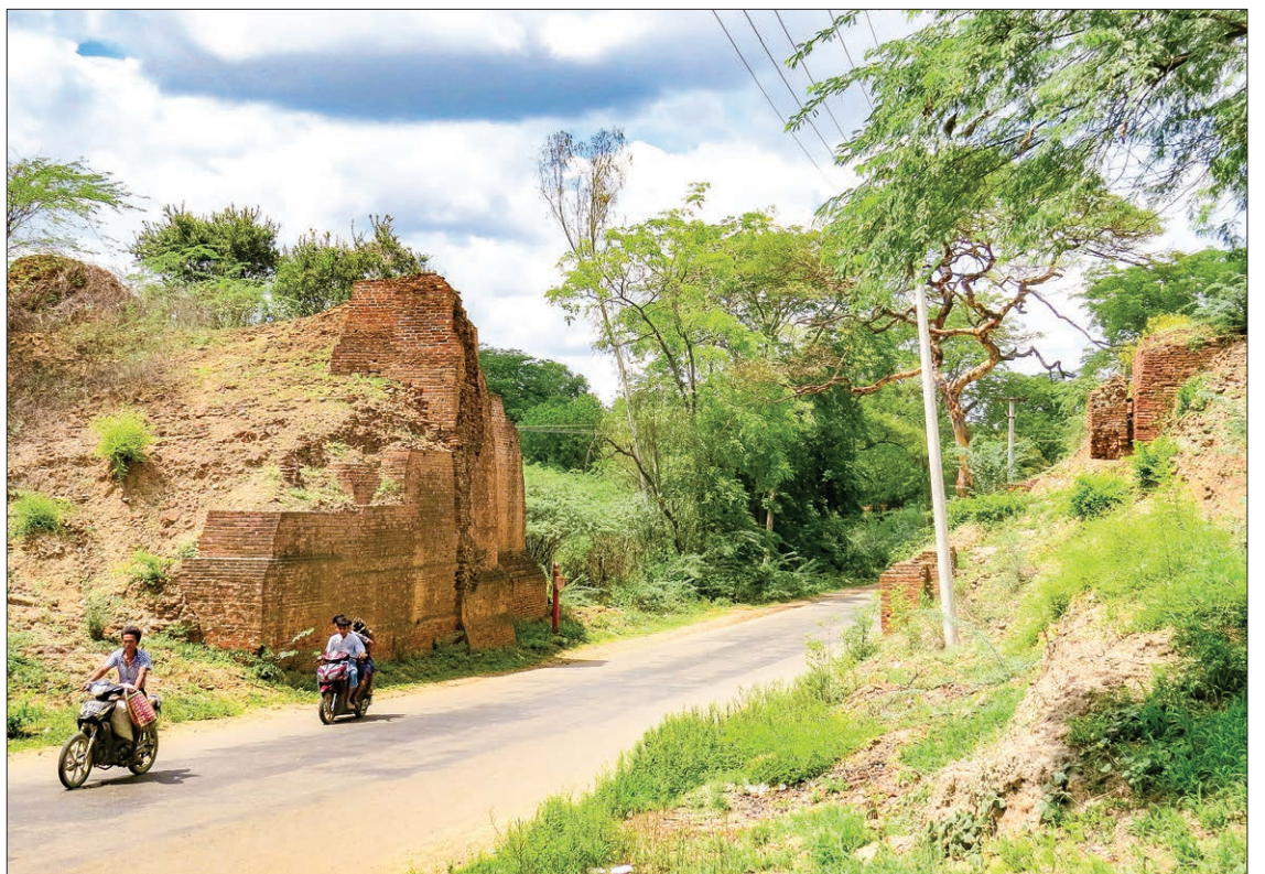
Ancient Pakhangyi city in Yesagyo Township has recorded over 300 religious buildings which need extensive preservation. PHOTO: ZAYYATU (MAGWAY)
