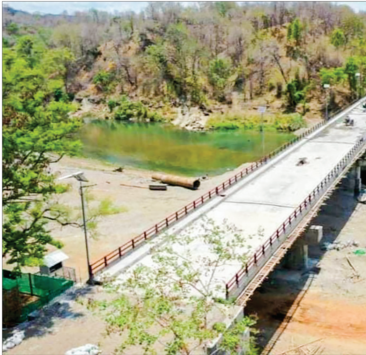
The bridge over the Mann Creek on the Pathein-Monywa Road in Minbu Township is set to be opened to traffic soon.
