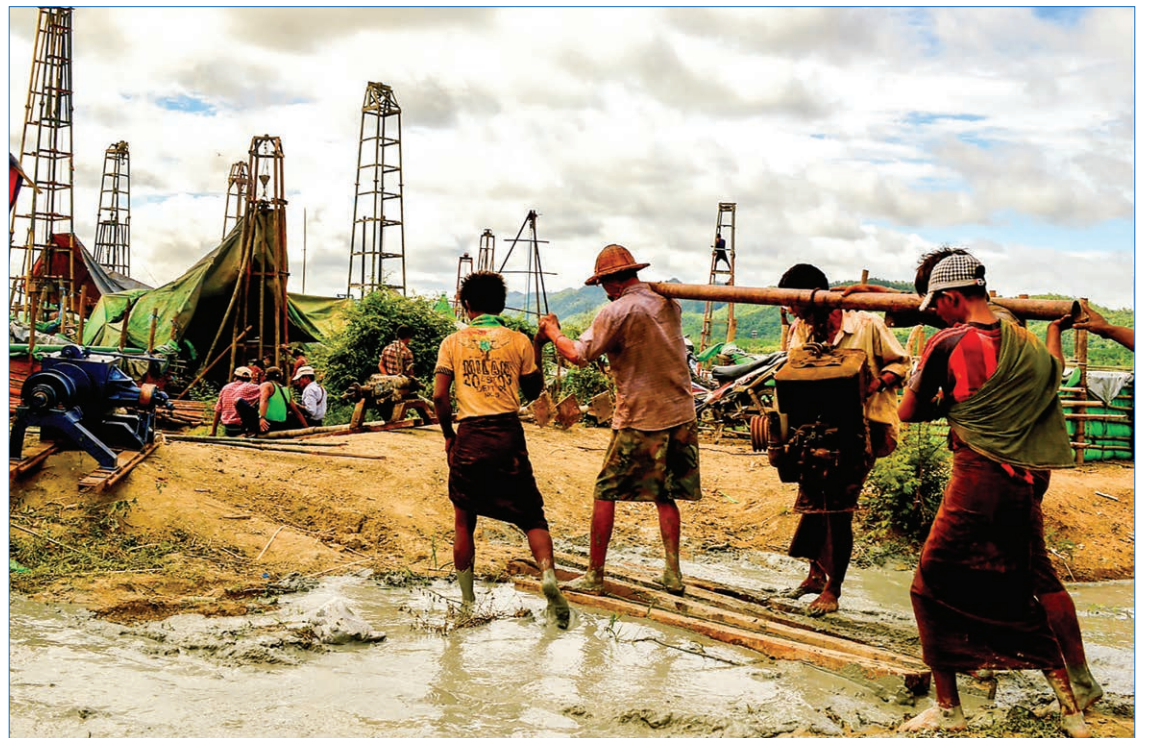
Workers carry an engine on their shoulder at a construction site in Kawthoung, Taninthayi Region on 31 July 2020. PHOTO: ZIN YAW AYE
