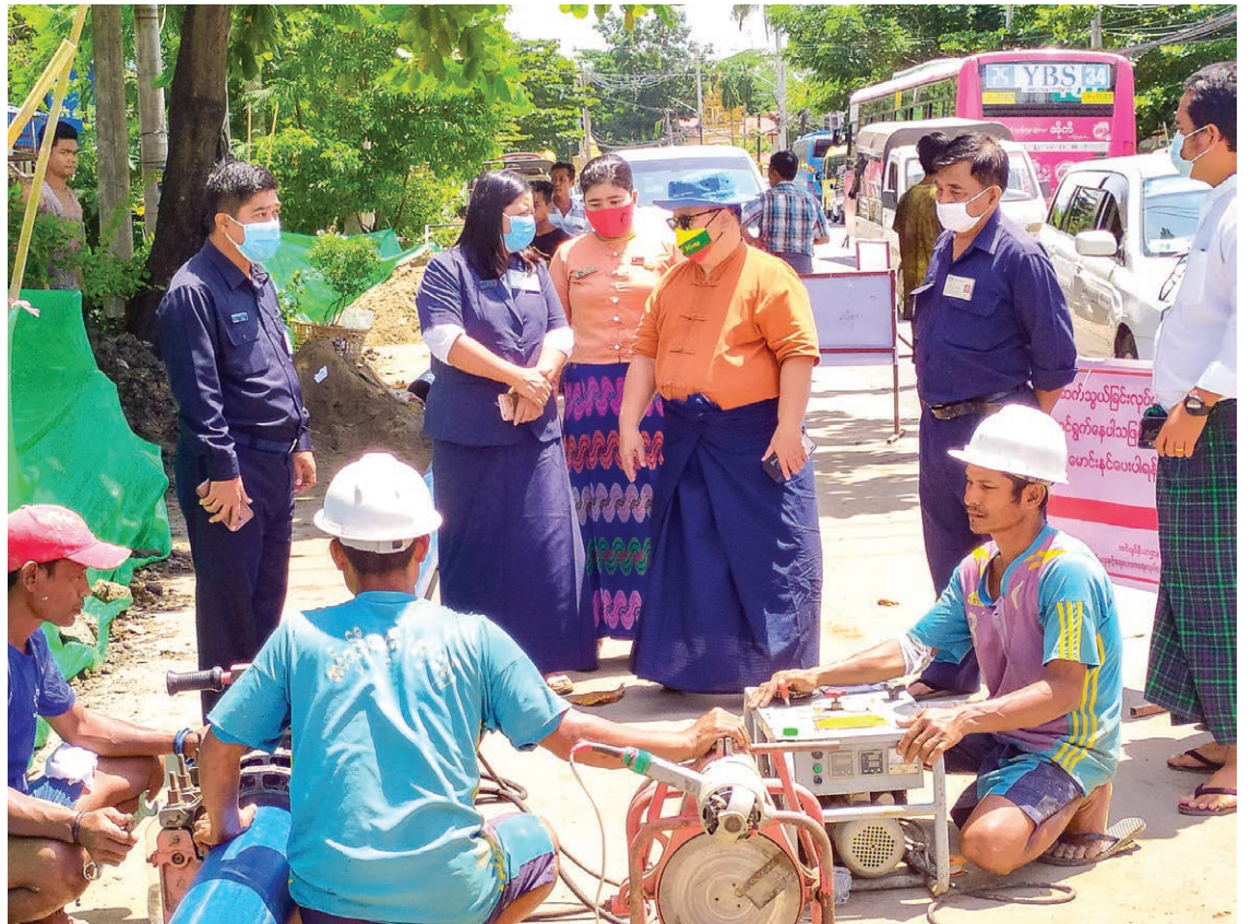
YCDC staff and officials inspect the replacement of water pipelines in Yangon on 26 July 2020. PHOTO: MYINT MAUNG SOE
