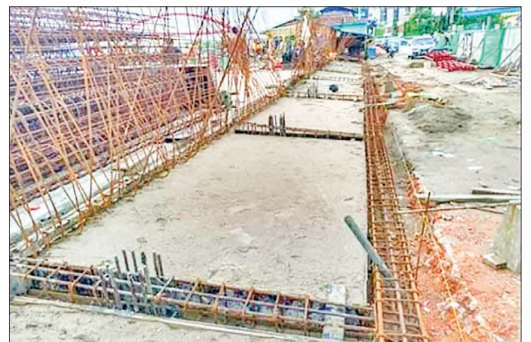
A line of concrete foundation is seen at Pathein jetty upgrade project i. PHOTO: MYINT MAUNG
