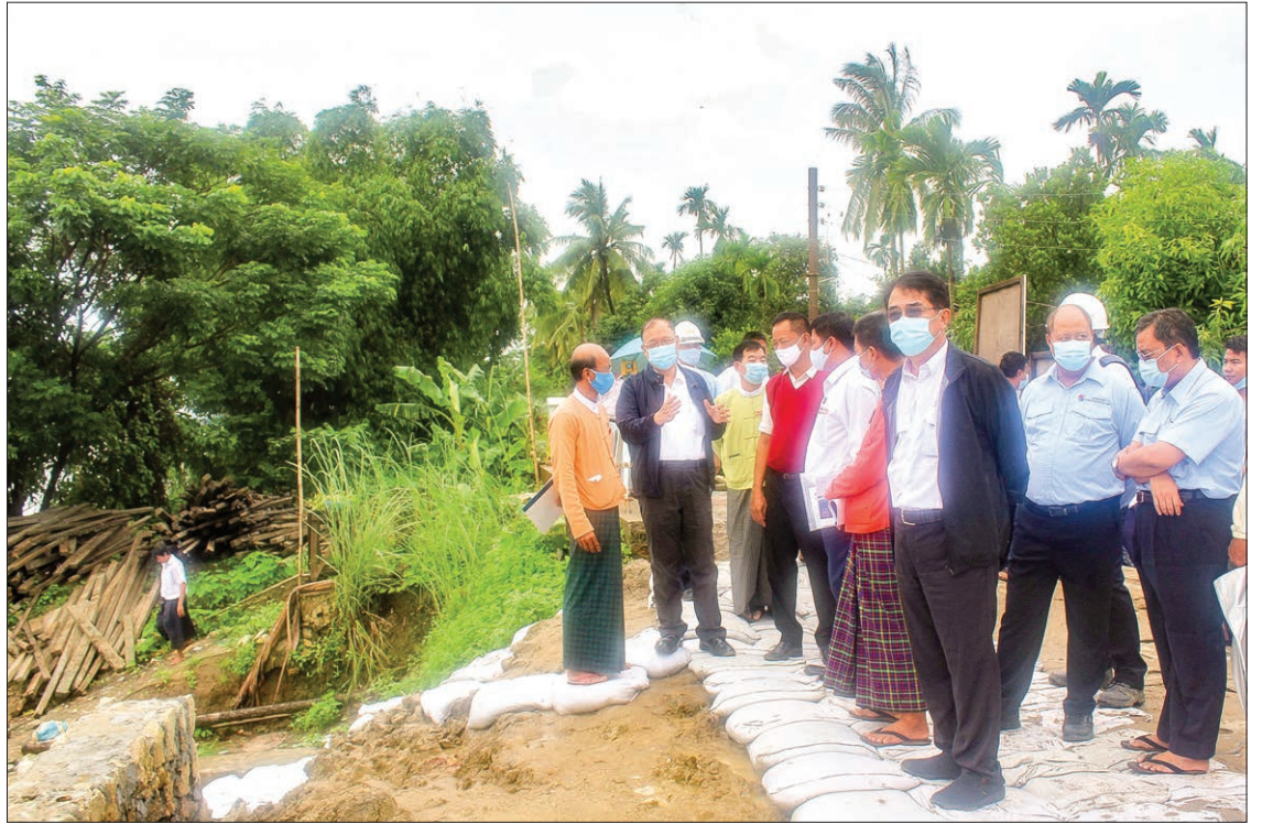
Union Minister U Thant Sin Maung and officials inspect Nyaungdon embankment project on 4 July 2020. PHOTO: MNA
