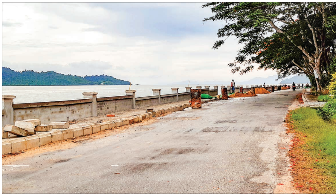
Circular road in Kawthoung, Taninthayi Region, is under renovation with railings and new pavement. PHOTO: KYAW SOE (KAWTHOUNG)
