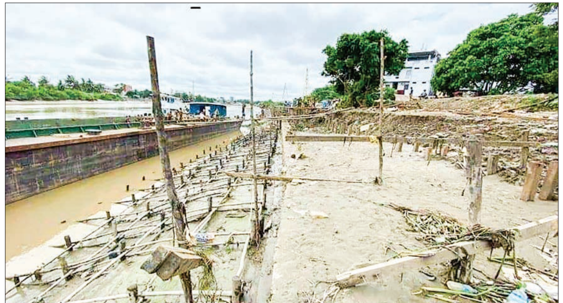
The erosion prevention work for the first five curves along the Nga Moe Yeik creek started in 2016.
