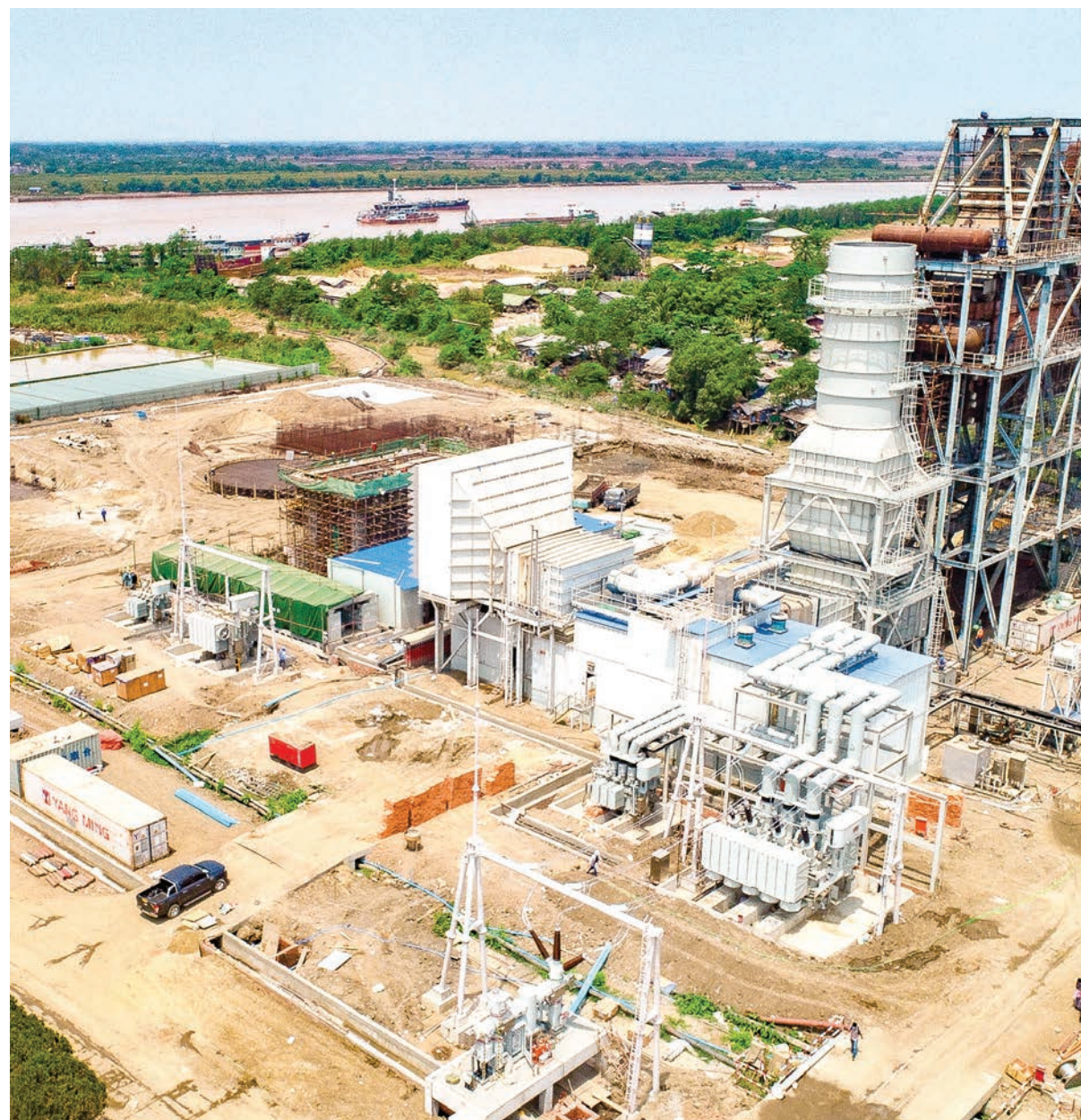
Ahlon power plant.
