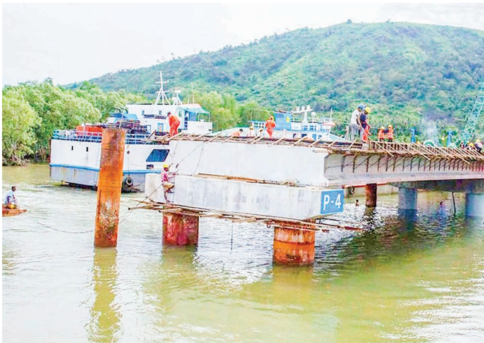
The Pulone Tone Tone Sea-crossing Bridge, the first of its kind in Myanmar is set to open to traffic soon. PHOTO: IPRD
