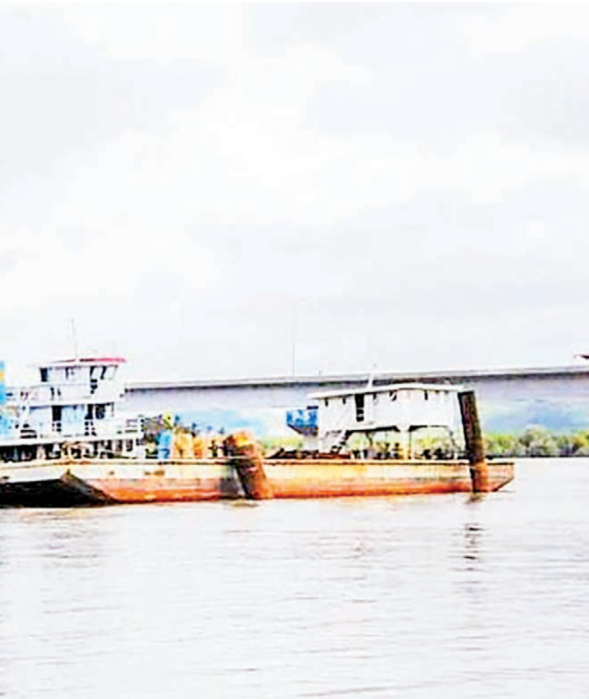
Tamote Lutlut Bridge is one of the major bridges under construction in Taninthayi Region and is 94 per cent complete. PHOTO: IPRD
