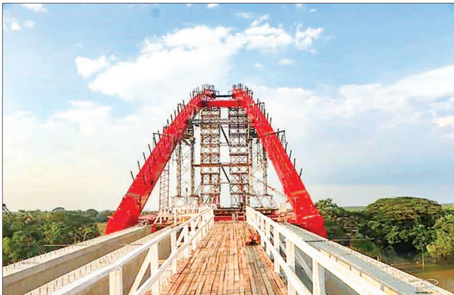
Sabel Gu (Attaran River Crossing Bridge) under construction on Kyaikmaraw-Sabel Gu-Koupanaw Road in Mon State.
