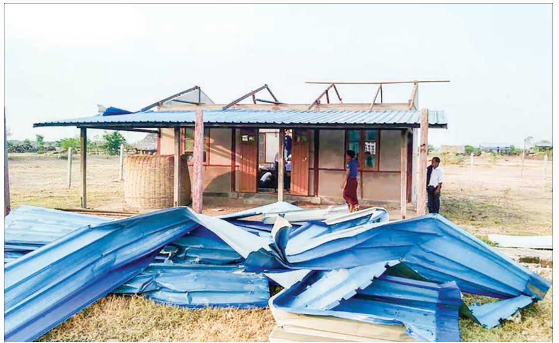
A building destroyed by a strong wind is seen in Kawlin, Sagaing Region. PHOTO: HMWE KYU ZIN
