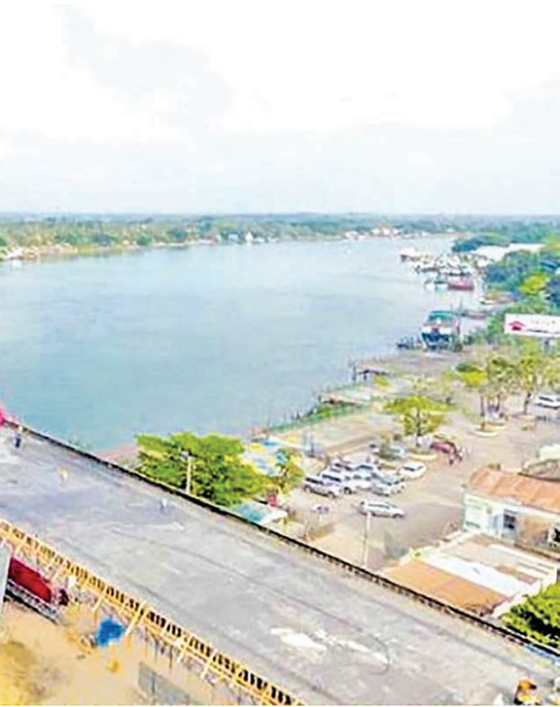
The Pathein Bridge-2 will become an important structure in Ayeyawady Region. PHOTO: IPRD
