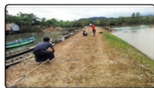
Repair of three cracks in Farmer Embankment in Taungnyo, Kyauk Phyu Township
