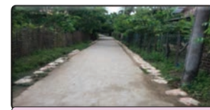
Upgrading into concrete road in Myitnarpyin Village, Aleichaung Village Tract, Ponnagyun Township
