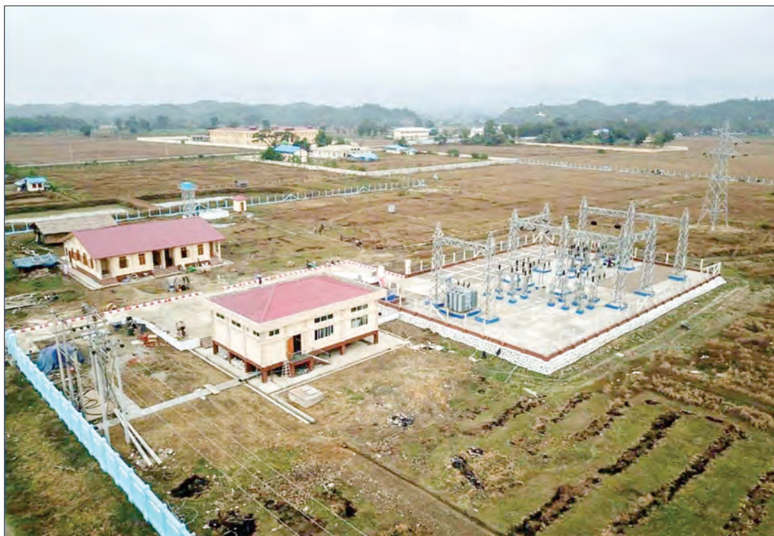
66/11 KV-5 MVA Sub-Power Station in Maungtaw.
