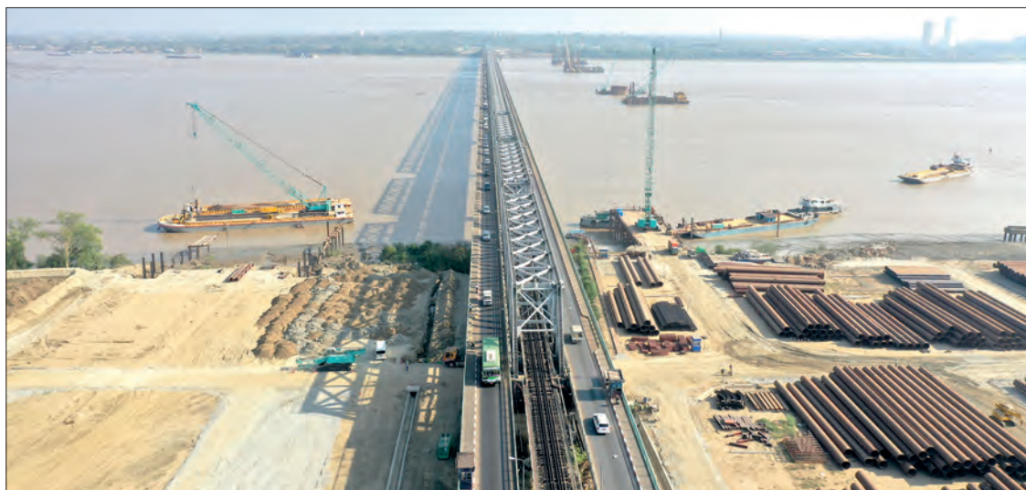
The Bago River-crossing Thanlyin Bridge No. 3 linking Yangon, Thanlyin and Thilawa Special Economic Zone is under construction.
