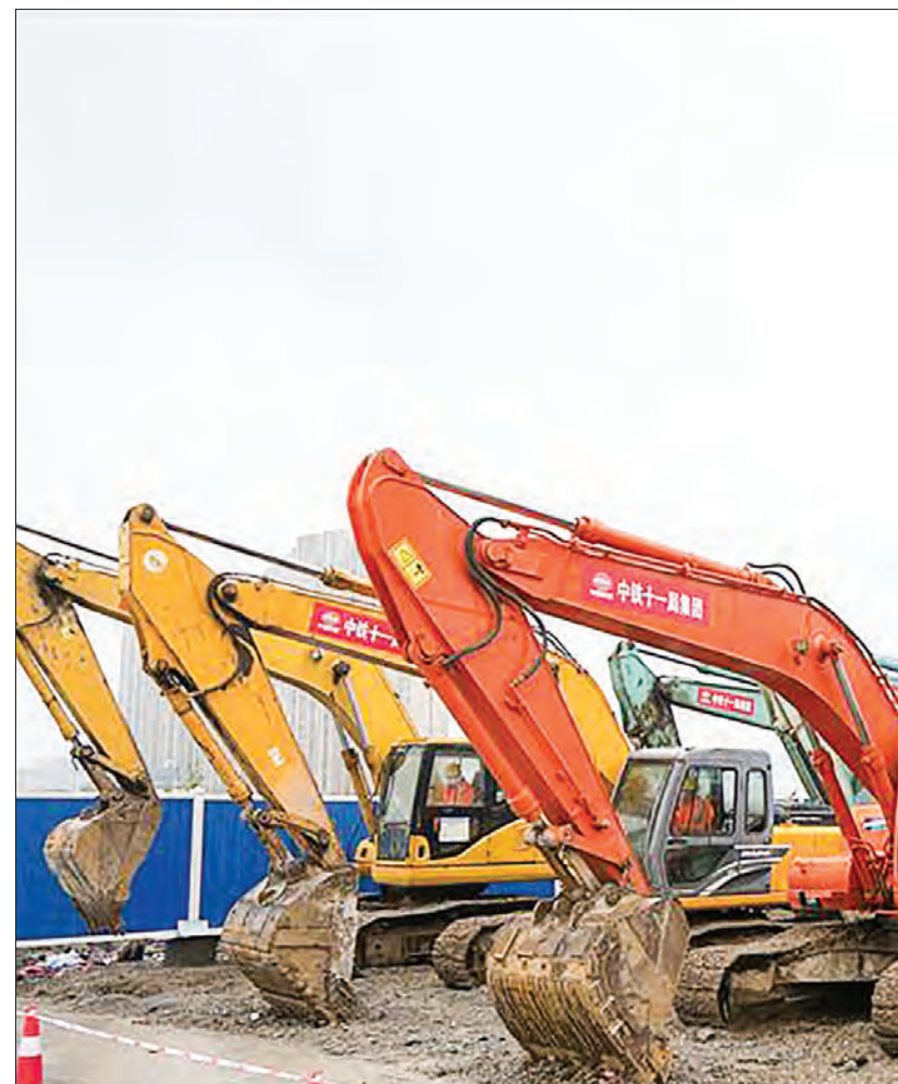
Labourers work at the construction site of a metro project in Wuhan, central China’s Hubei Province on 30 March, 2020. Wuhan’s 12 metro projects under construction resumed work up to Monday. PHOTO: XINHUA
