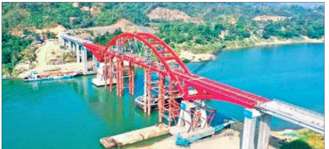
The Kaladan River crossing bridge in Chin State's Paletwa Township is set to open to traffic soon. (PHOTO: IPRD)
