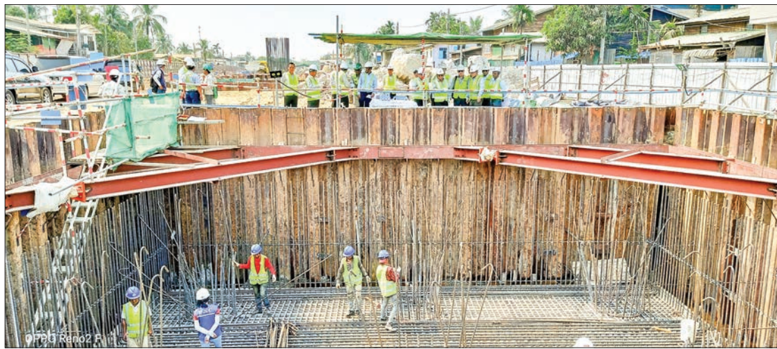
Union Minister U Han Zaw and party inspecting the construction project of Korea-Myanmar Friendship Bridge (Dala) in Yangon yesterday. PHOTO: MNA
