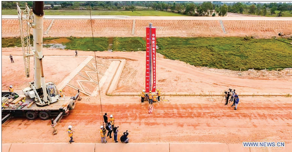
Workers plant the first engineering pole at the construction site of the China-Laos railway project in Vientiane, Laos, March 15, 2020. PHOTO: XINHUA
