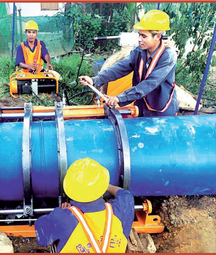
Municipal workers check to assure proper maintenance of water pipe.
