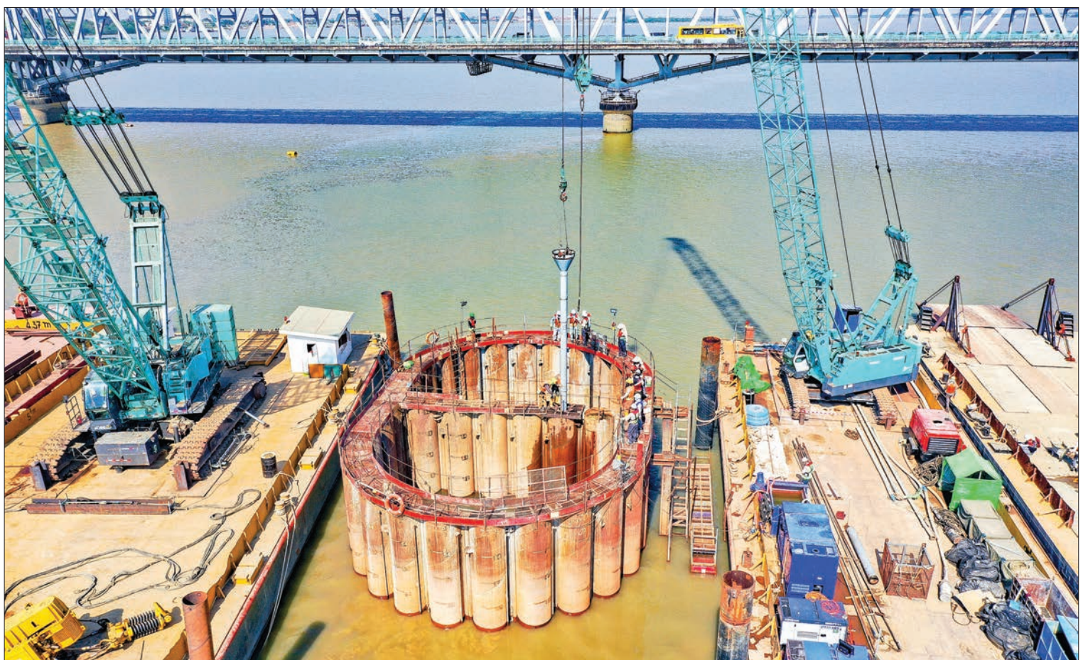
The Bago River-crossing Thanlyin Bridge No. 3 linking Yangon, Thanlyin and Thilawa Special Economic Zone is under construction. PHOTO: MNA
