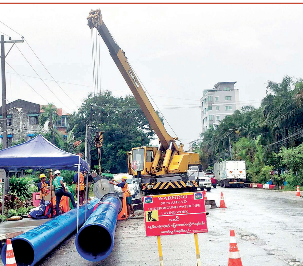
Municipal workers are in process of laying water pipelines to supply drinking water in Yangon municipality.
