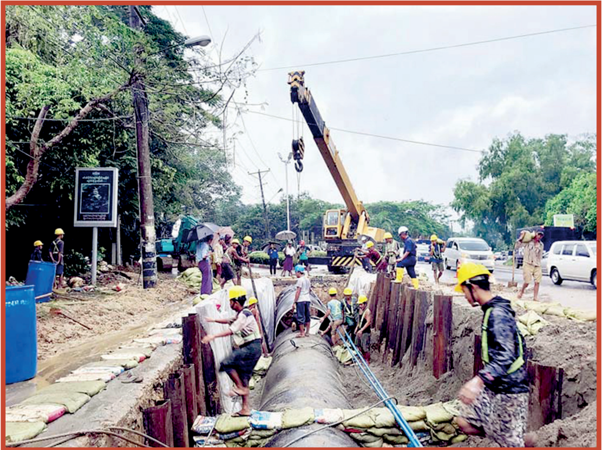
Municipal workers are replacing old pipelines with new ones in Yangon municipality.
