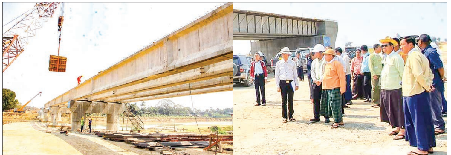
Bago Region Chief Minister U Win Thein visits the construction of Sittaung river crossing bridge (Yedashe). PHOTO: HEIN HTET (BAGO)
