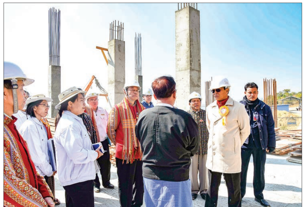
Vice President U Henry Van Thio visits the construction site of the three-storey Chin State High Court. PHOTO: MNA
