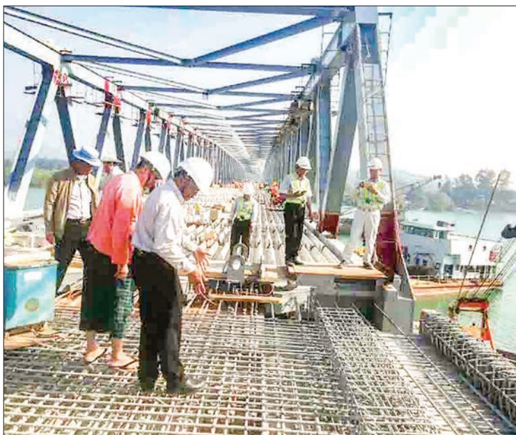
Rakhine State Chief Minister U Nyi Pu, Minister for Electricity, Industry, Roads and Transport U Aung Kyaw Zan and district and township level officials inspecting the construction of Kinkaung bridge in Kyaukpyu, Rakhine State yesterday. PHOTO: MNA
