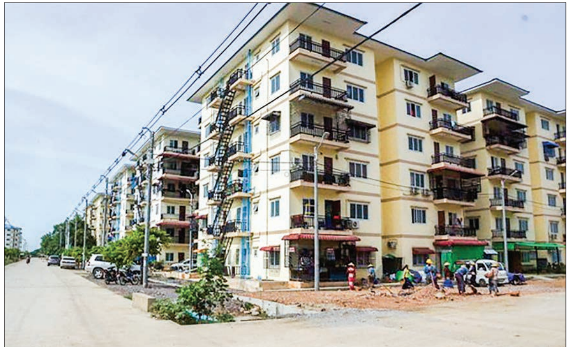
The Myayee Nanda apartments are being built for retired government servants, private companies' staff and the general public. PHOTO:THAN ZAW MIN (IPRD)
