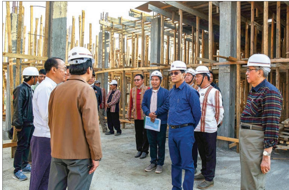
Vice President U Henry Van Thio inspects the construction of Thantlang People's Hospital. PHOTO:MNA
