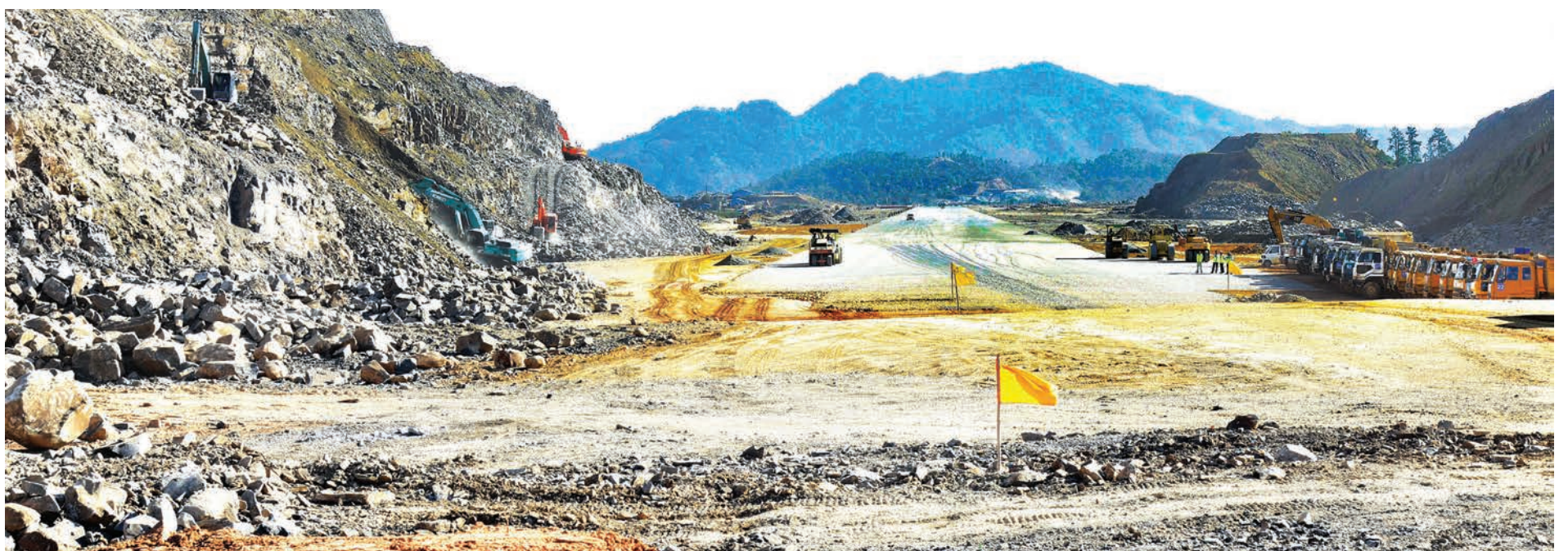
Vice President U Henry Van Thio inspects the construction of the Surbung Airport in Falam Township, Chin State. PHOTO: MNA
