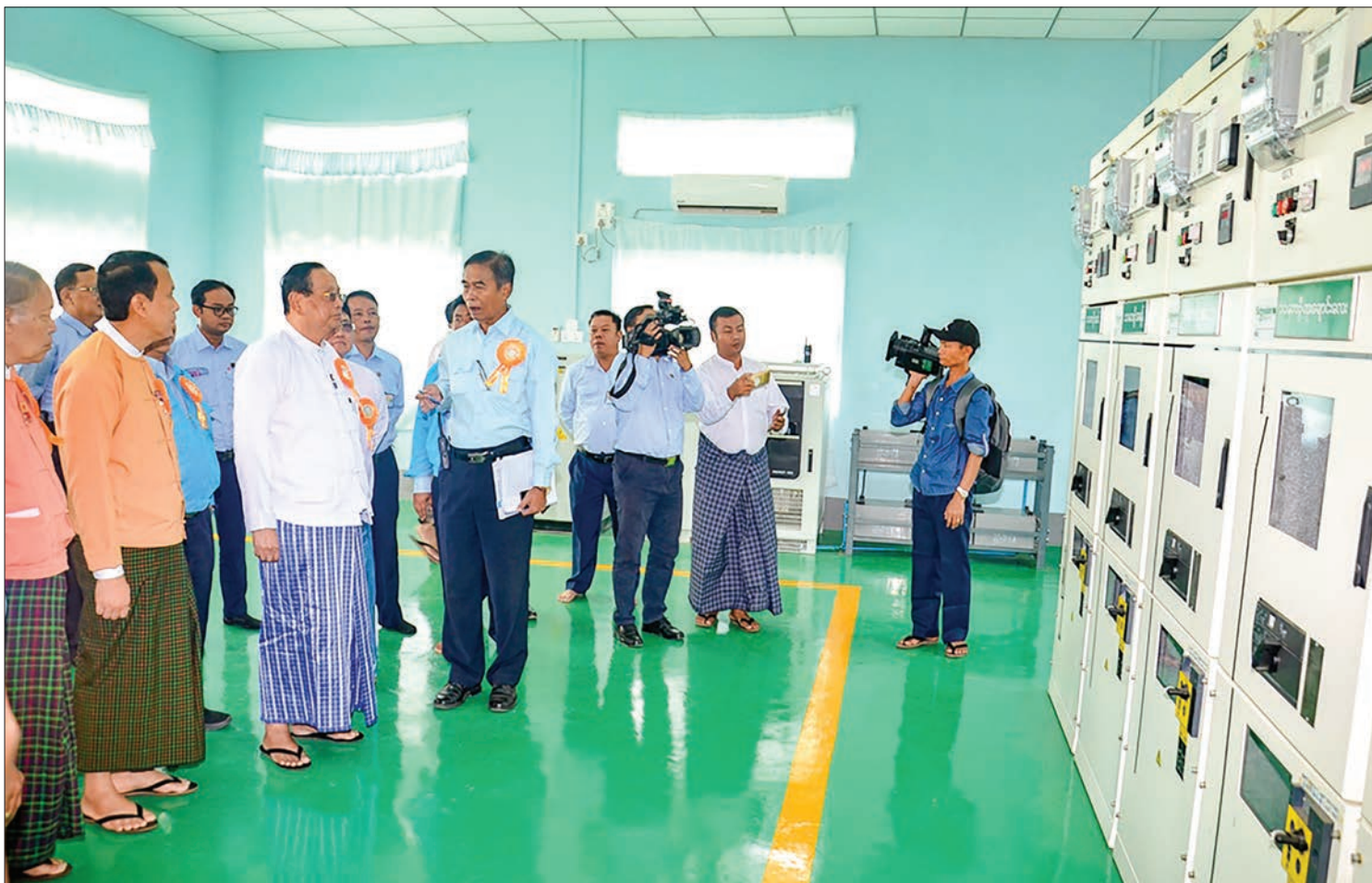
Union Minister U Win Khaing and Yangon Region Chief Minister U Phyo Min Thein visit the 33/11 kV-5 MVA substation in Twantay Township yesterday. PHOTO: MNA
