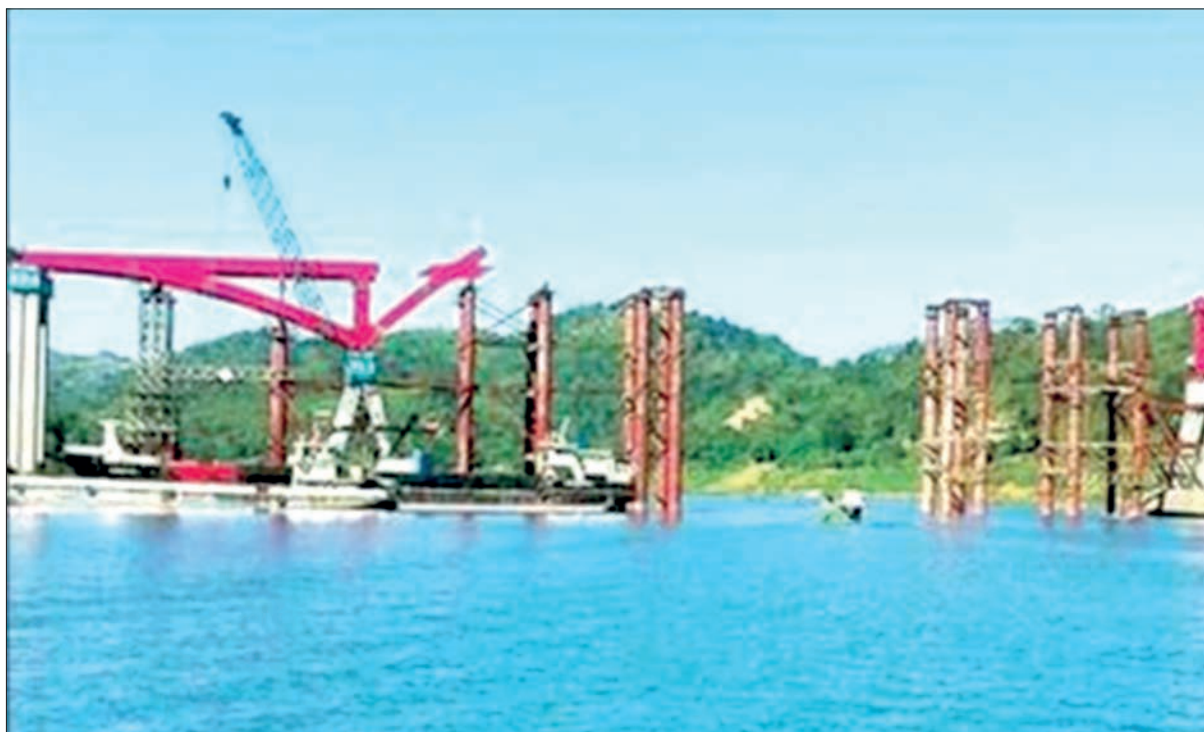
The Kaladan River Crossing Bridge Project is slated for completion by the end of March this year. PHOTO: MG MG KYAWT
