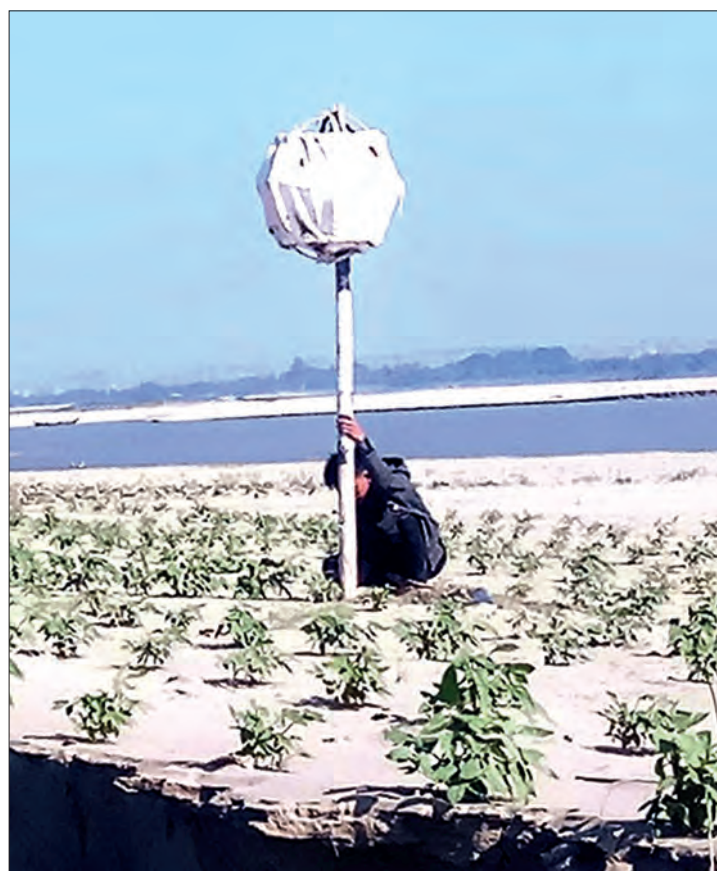
An official installing a navigational aid near the Ayeyawady River in Magway. PHOTO: ZAYYARTU (MAGWAY)
