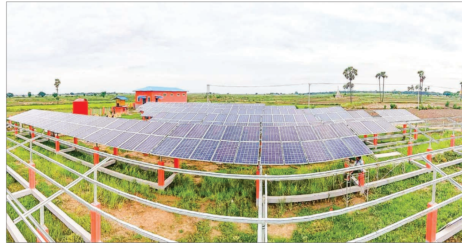
Eight villages between Ayeyawady and Chindwin rivers in Yasogy Township get access to solar power last year. PHOTO: THAN LWIN (MAGWAY)
