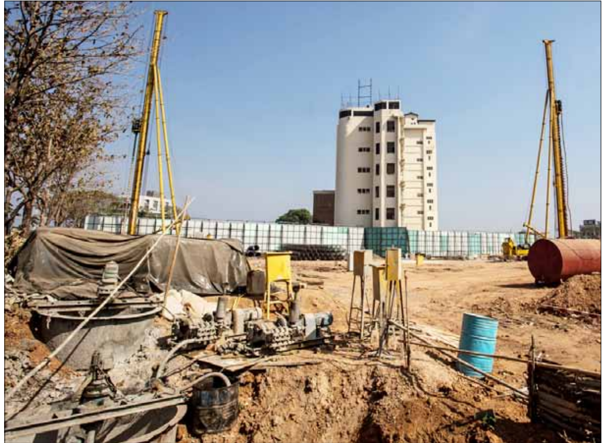
The site of the Polo Club Asia Residence building, with the former National Library at centre. Photo: Zarni Phyo
